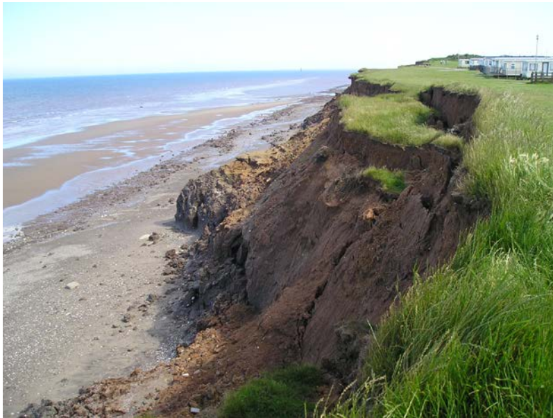
Rotational failure of till cliff, Aldbrough, Holderness, 2005.
